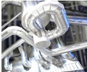
Heating, ventilation and air conditioning
